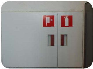
Storage space for fire-extinguisher
